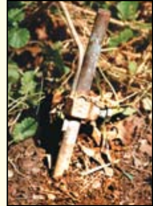
Grounding rod in the earth.
